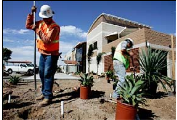
LAURA EMBRY / Union-Tribune Landscapers Artemio Rodriguez (left) and Jesus Marquez dug holes for plants surrounding the operations center at the southern tip of the South Bay Expressway in Chula Vista.
