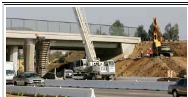
Frank Bellino / The Press-Enterprises Construction crews work on the Los Alamos Road overpass and offramps for Interstate 215 in Murrieta.
